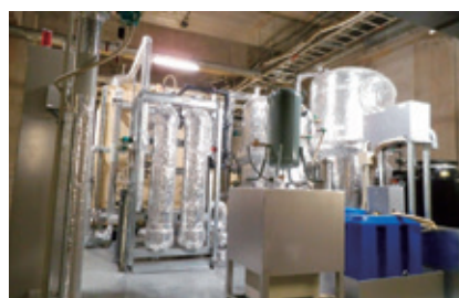
Groundwater filtration system at Nagoya PARCO
